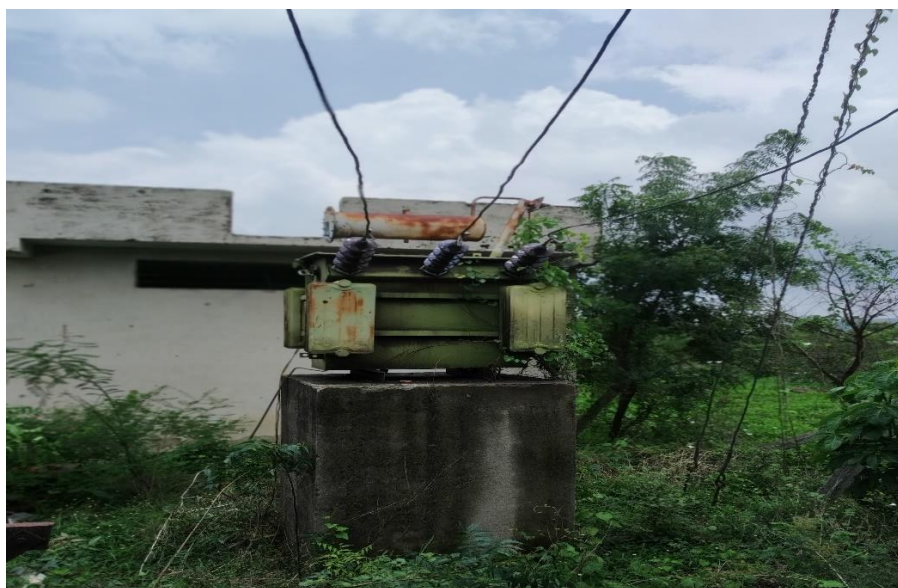
Fig. 2.1 - Transformer in college
