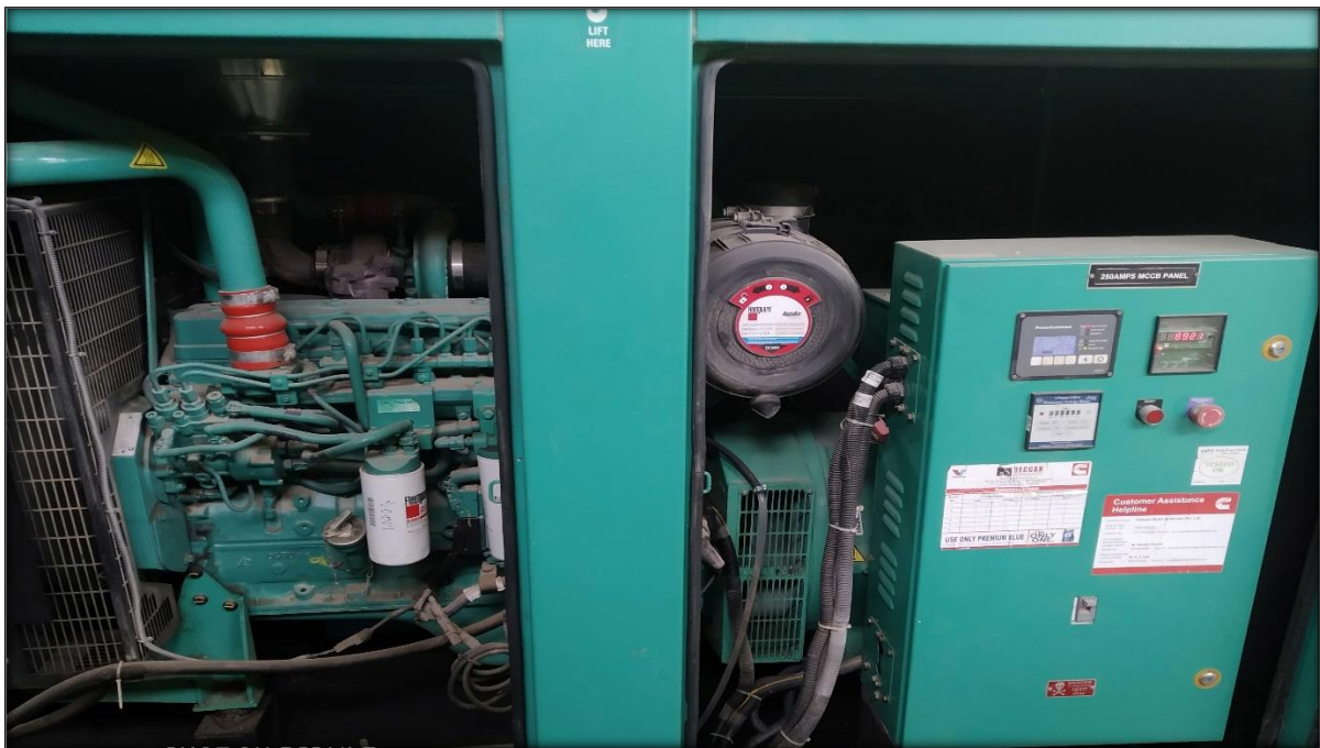
Figure 2.4: - DG set in Institute
