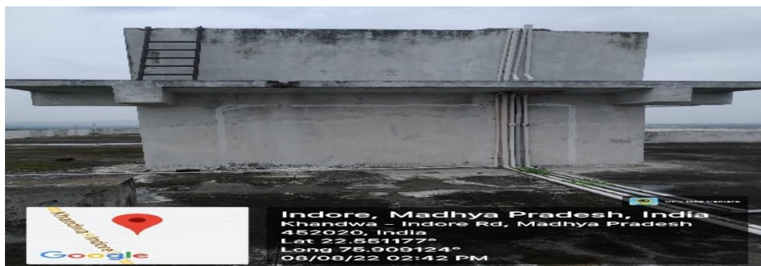
Fig :2.3 Water storage tank in institute
