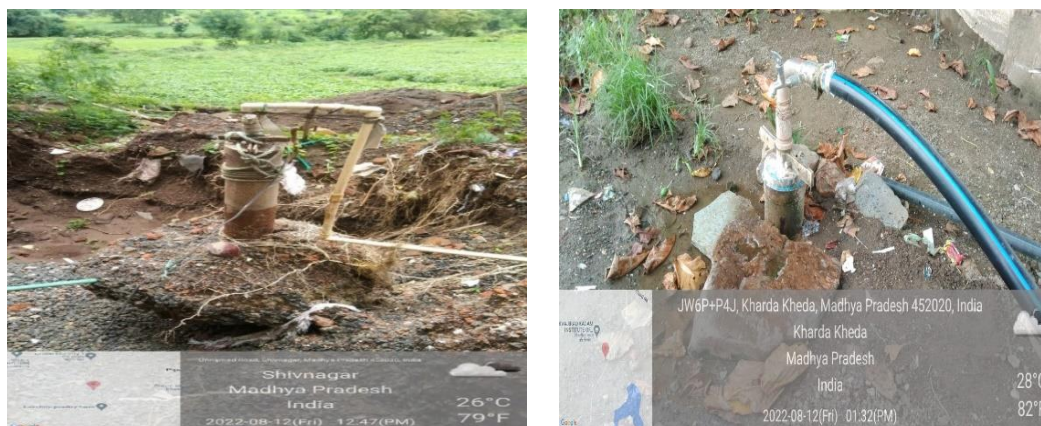
Fig :2.1 Fresh water supply from borewell of college campus
